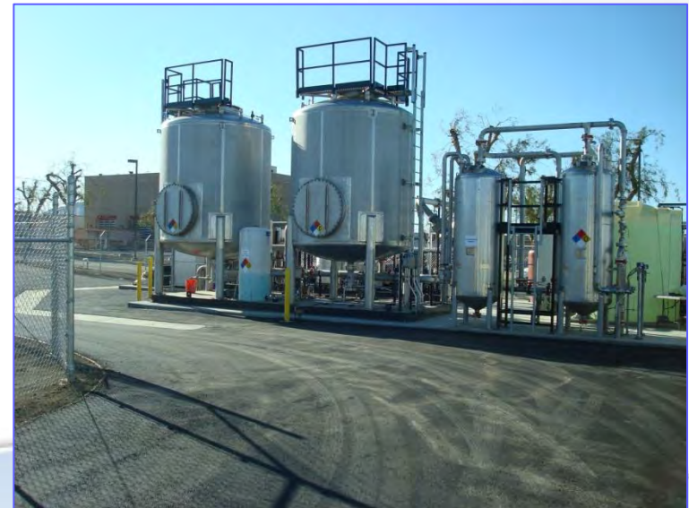
Digester Gas Treatment System, EMWD-Moreno Valley, CA
