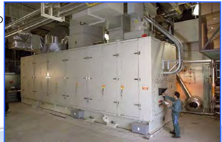
3.5 MW gas turbine Cogeneration System
