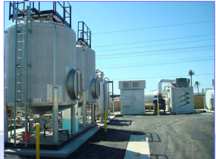
250-kW Digester Gas Fueled Fuel Cells, EMWD-Moreno Valley, CA
